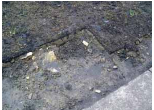
Surface water running onto adjacent paving
